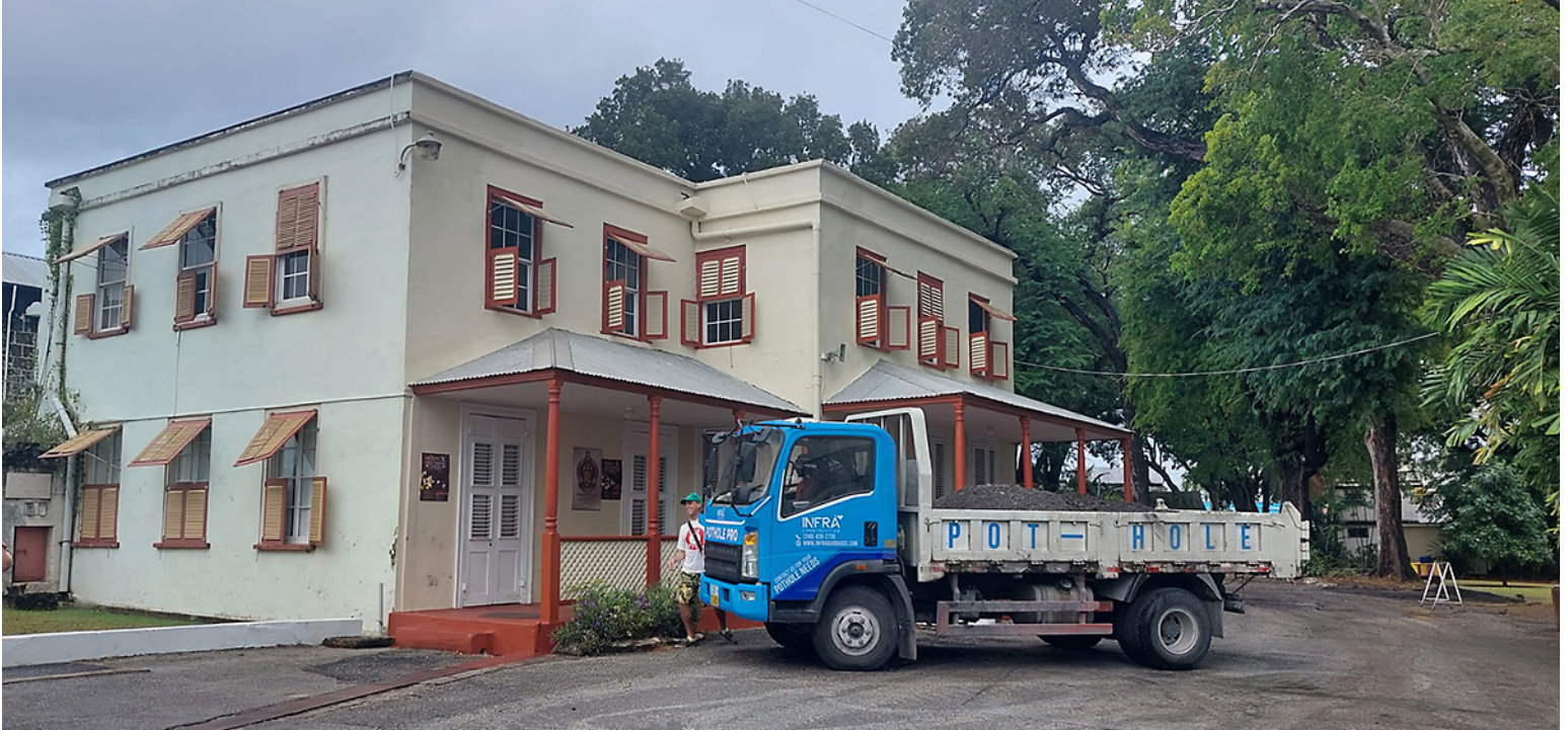
Hamilton "Hammie" Hinds on-site at Harrison College in early March 2025. The INFRA Construction team were busy patching potholes!
